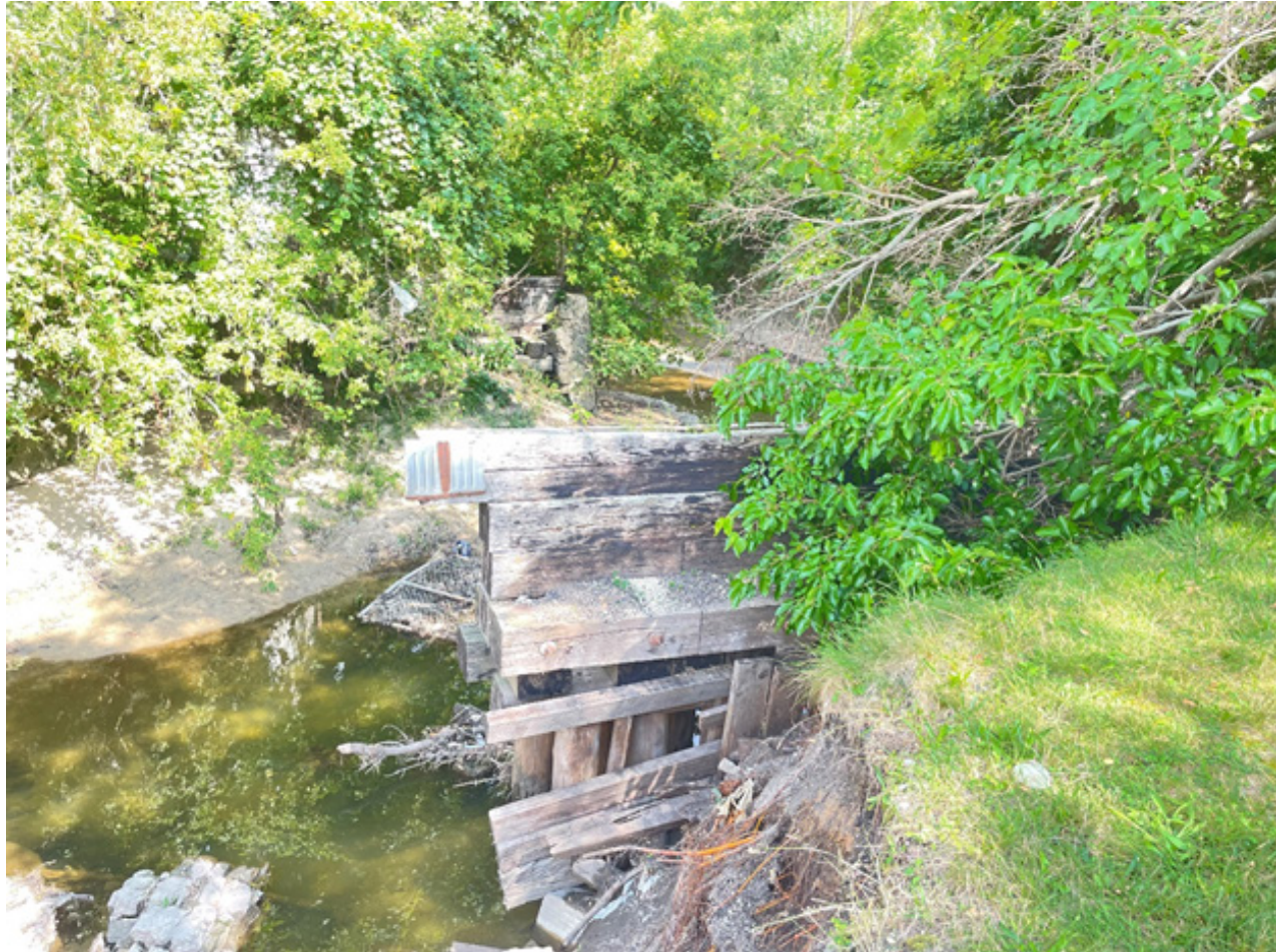
Bank erosion and remnants of the former railroad bridge abutment protruding into Keith Creek upstream of 18th Street.
