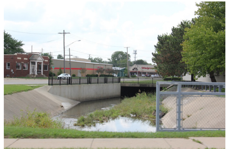
The existing Charles Street box culvert showing sedimentation and plant growth in the concrete channel. The culvert is currently being evaluated by the City for replacement to increase conveyance capacity.
